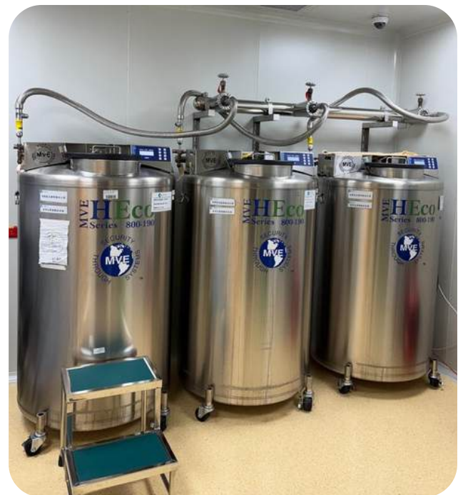
Liquid nitrogen storage tanks utilized for long-term WJ-MSC storage
